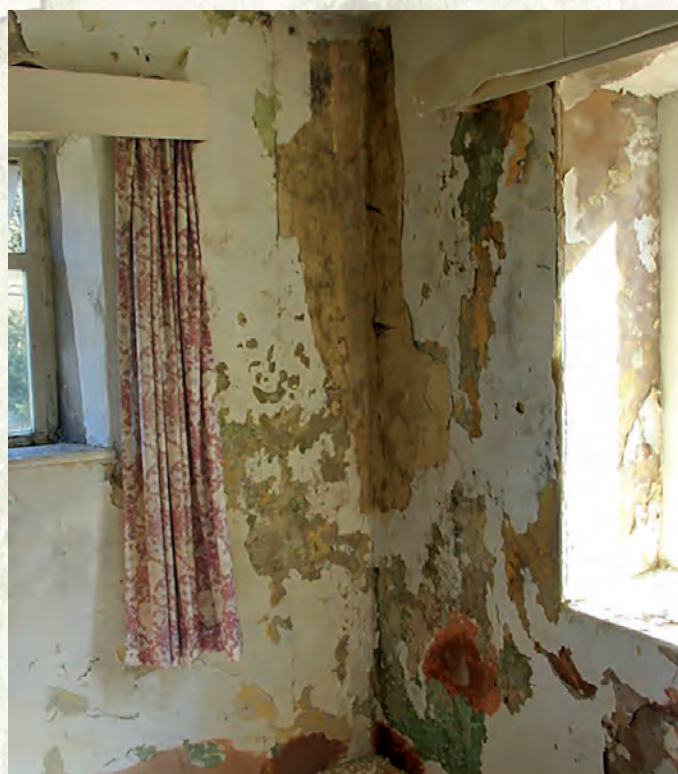
Interior of first floor damp walls before removal of cementitious materials prior to wood fibre insulation and lime plaster
