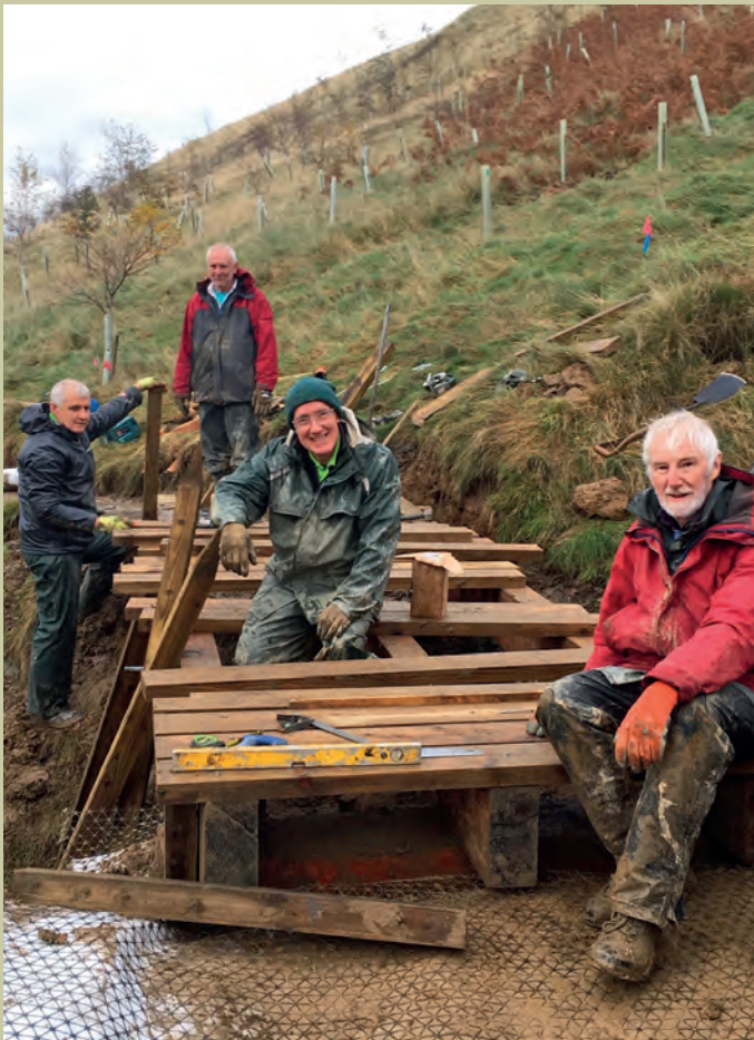
Dales volunteers installing a new footbridge on a path being created by agreement with the Lonsdale estate on Tebay Fell.
